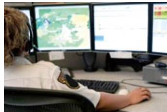
Multiple Control Displays
