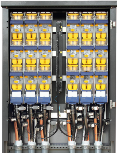
SGU installed in a standard steel cabinet
